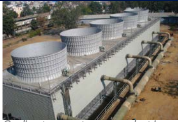
Cooling towers at a power plant in India
