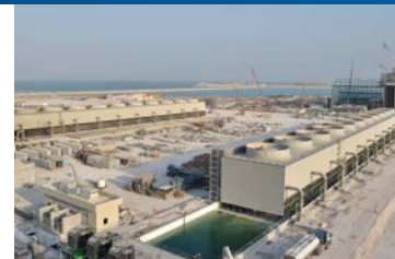
850 MW sea water cooling towers at a combined cycle power plant in Qatar
