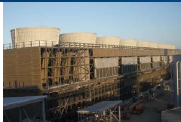
Wet/dry cooling tower serving 600 MW power plant
