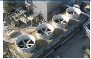
Wooden cooling tower for a 220 MW power plant
