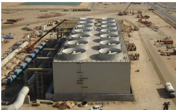
FRP cooling towers at a refining and petrochem complex in Saudi Arabia
