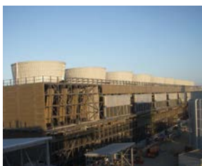
Hybrid installation in the U.S.
