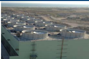
FRP cooling towers – 900 MW power plant in Turkey
