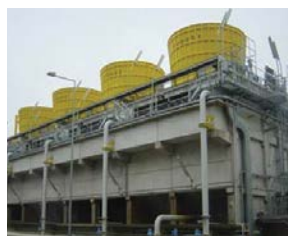
Hybrid installation in Italy
