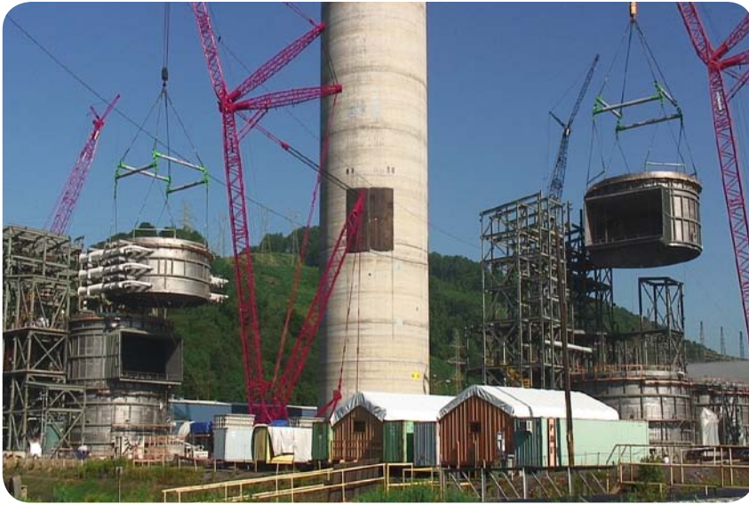
Dual wet FGD lift, June 2008.
