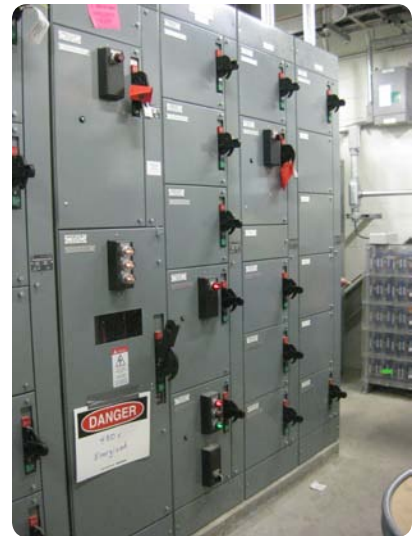
SCR motor control centers.
