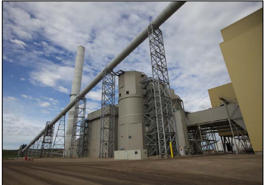
Spray dryer absorbers and pulse jet fabric filter for Keephills Unit 3.
