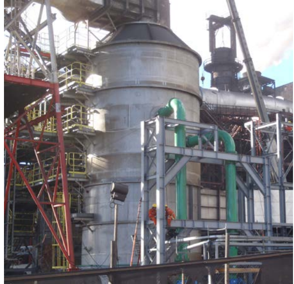
Wet scrubber for \text{SO}_x control.
