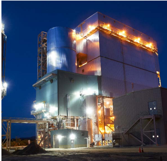
Circulating dry scrubber with fabric filter for \text{SO}_x and particulate control.
