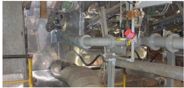
New pneumatic limestone injection system.
