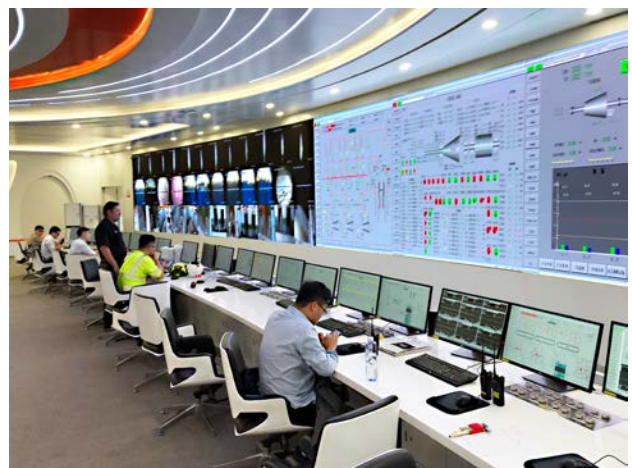
Modern control room at Shenzhen East.
