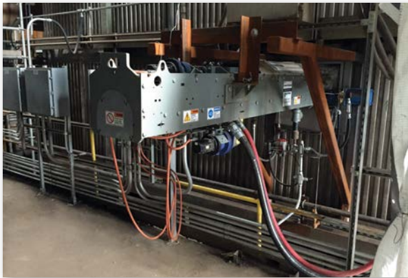
HydroJet-R system installation (top cover plate removed for maintenance)
