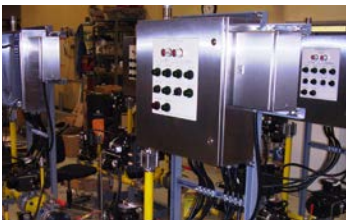
Burner/ignitor valve train with local control panel
