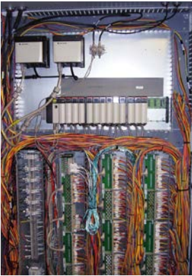
Burner management system control cabinet wiring
