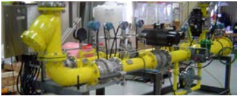
Main gas header valve train
