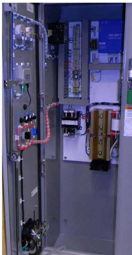
Typical single-phase AVC cabinet
