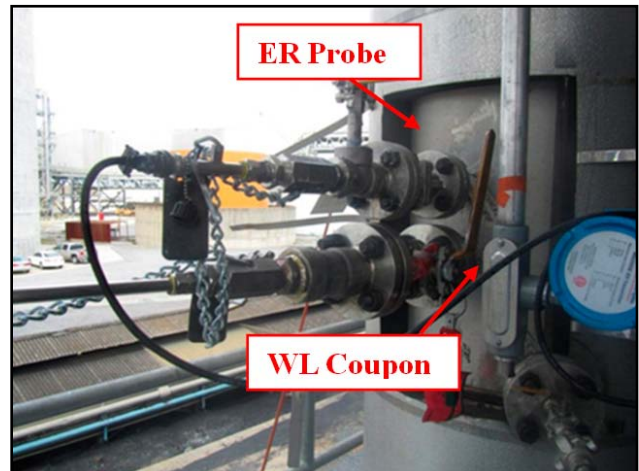
Fig. 4 Typical corrosion measurement location.
