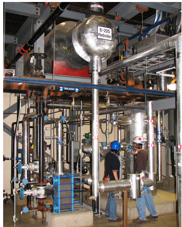
Fig. 6 B&W PGG's RSAT pilot plant.
