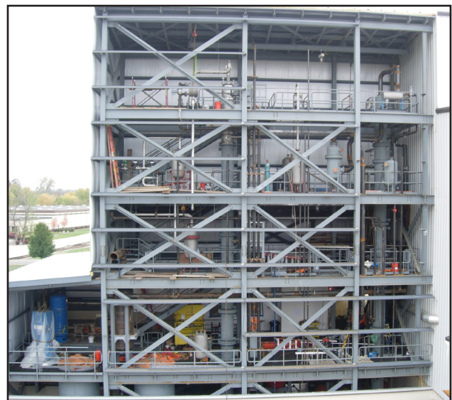
Fig. 1 B&W PGG's post-combustion pilot test facility.
