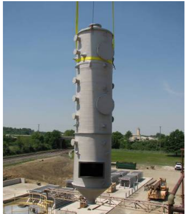
Fig. 6 Wet FGD absorber tower.
