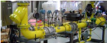
Main gas header valve train
