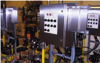
Burner/ignitor valve train with local control panel
