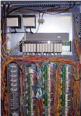
Burner management system control cabinet wiring
