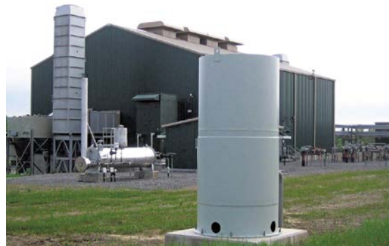
Turbine exhaust silencer and vent blow-down silencer at a gas compression station.
