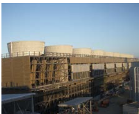
Hybrid installation in the U.S.
