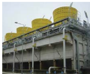
Hybrid installation in Italy
