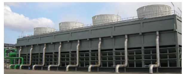
Concrete cooling towers
