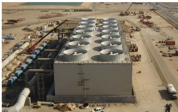
FRP cooling towers at a refining and petrochem complex in Saudi Arabia
