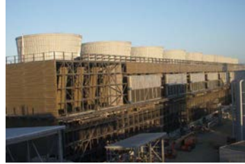
Wet/dry cooling tower serving 600 MW power plant
