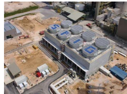
Noise-abated cooling towers at an 800 MW power plant
