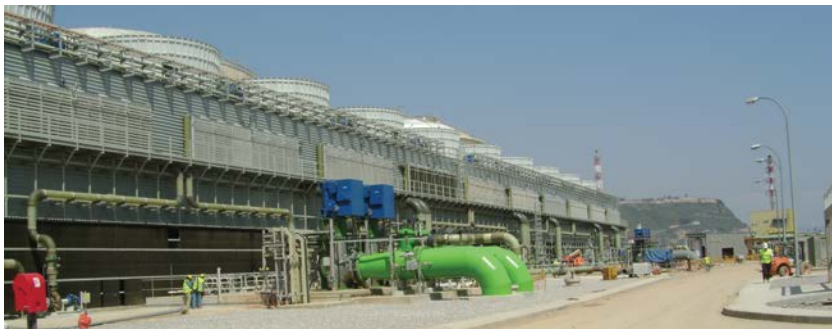
Sea water cooling tower, 2 x 425 MW combined cycle power plant
