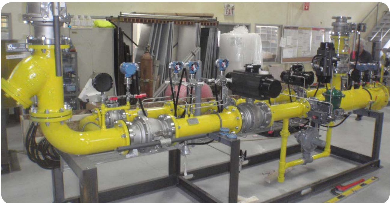
Shop-assembled main gas header valve train.
