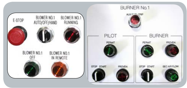
Cooling air blower and igniter burner controls.
