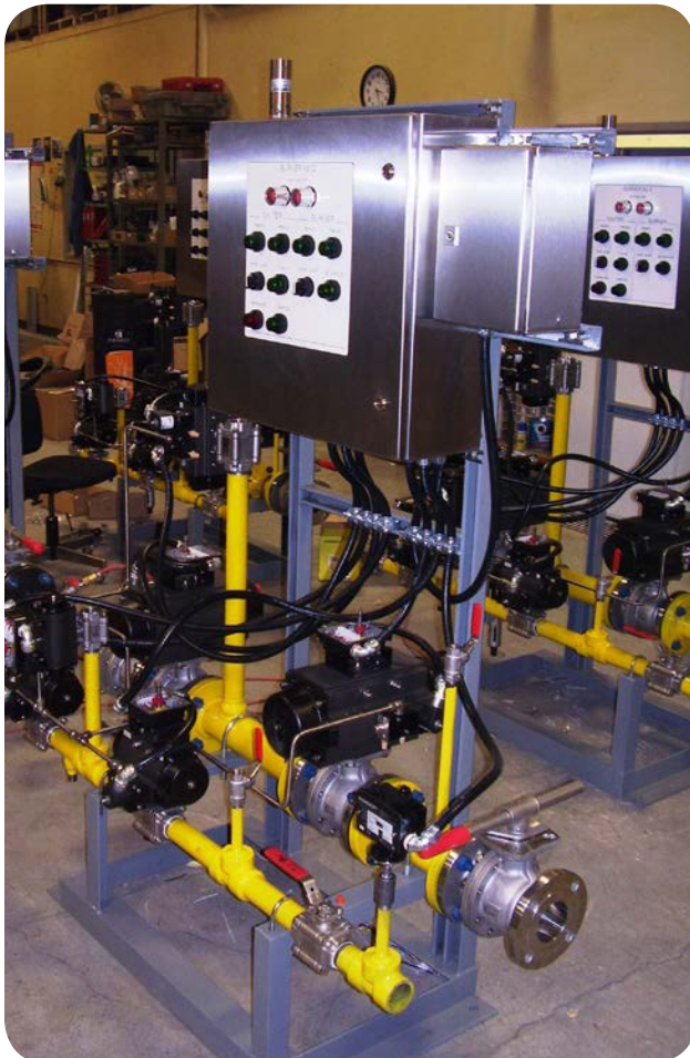
Burner/igniter valve train with local control panel.
