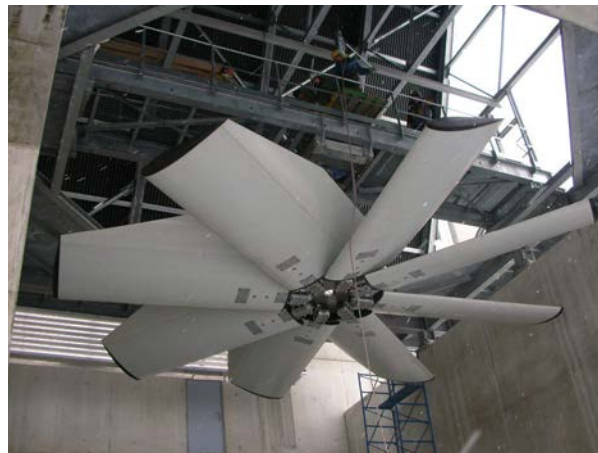
Air-cooled condenser service
