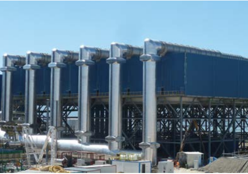
Air-cooled condensers for an 850 MW combined cycle power plant
