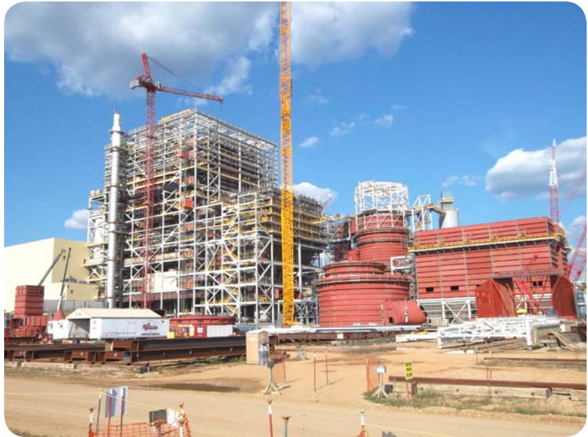
The 600 MW John W. Turk, Jr. Power Plant features advanced, ultra-supercritical boiler clean coal combustion technology.
