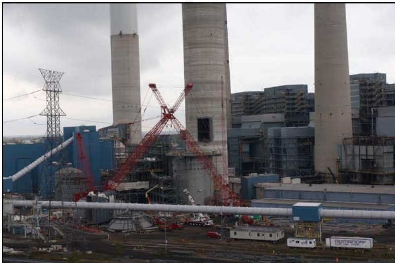
BWCC provided construction services for all B&W PGG-supplied wet FGD system equipment at the Monroe power plant.
