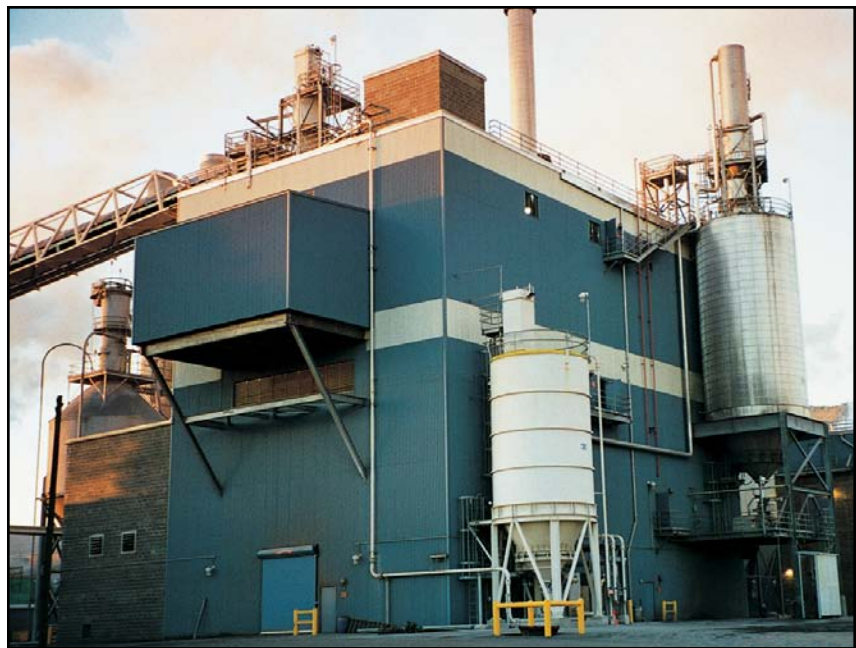
This BFB unit is now burning 100% of the sludge produced at the mill and is operating 25% above the original rated capacity.
