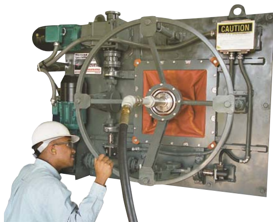
Fig. 2 Diamond Power Specialty Company Hydrojet® boiler cleaning system.
