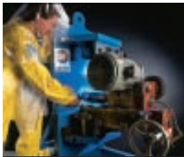
Extensive mockup training and testing ensures successful site execution, consistent with ALARA goals.
