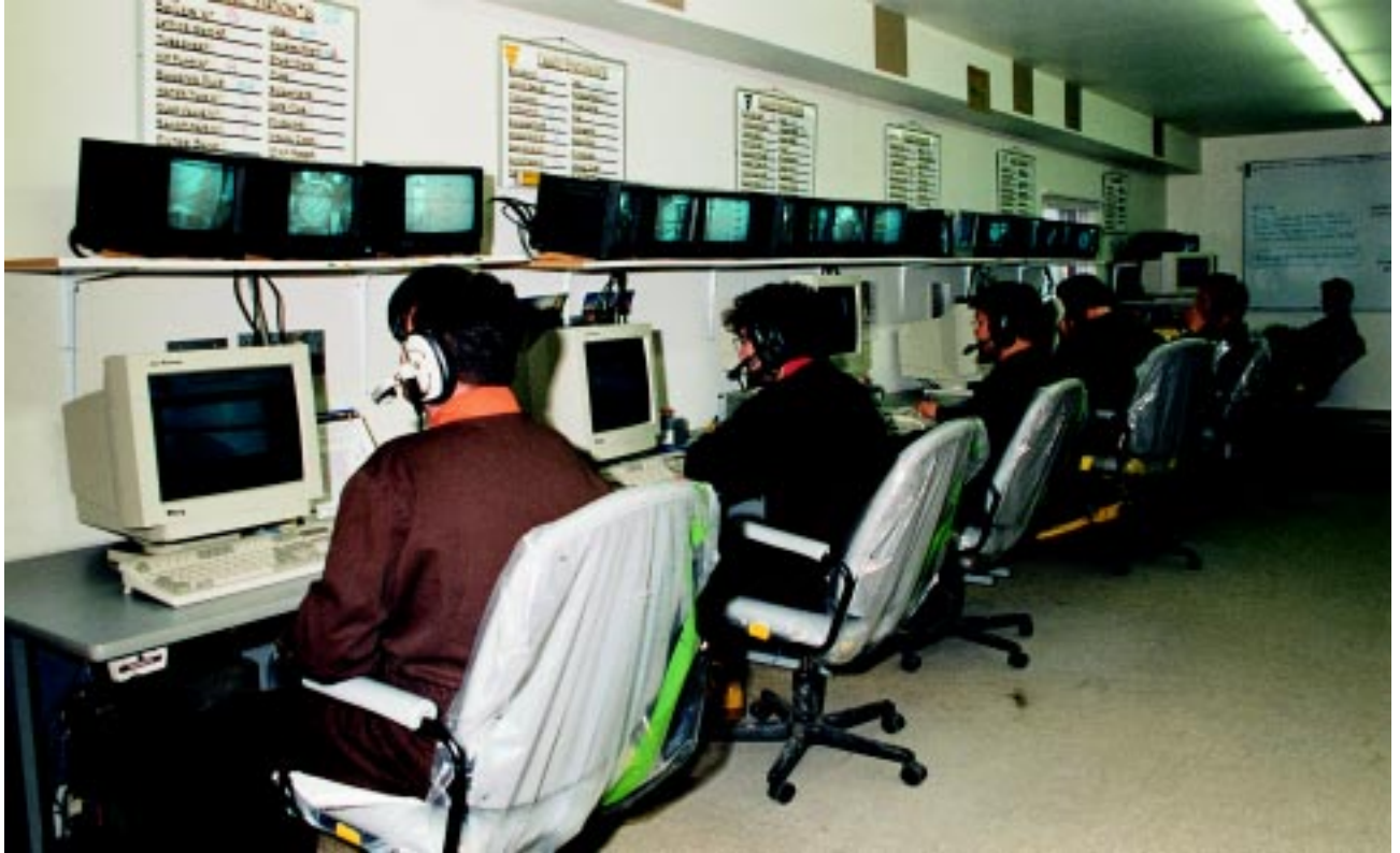
Waterlancing remote control work stations at Pickering NGS where Babcock & Wilcox deployed 12 waterlance systems in parallel
