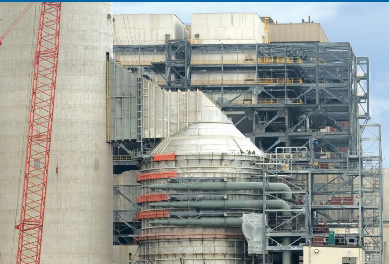
Current B&W designs are achieving 99% SO 2 removal with system availability greater than 99.5%.
