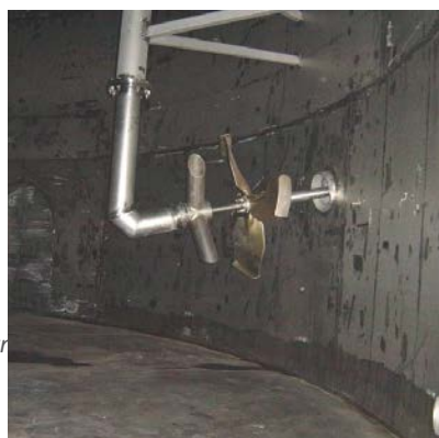
Multiple side-entering agitators on B&W's absorber tower provide uniform slurry mixing.
