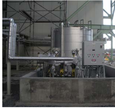
The Absorption Plus (Hg) ™ system utilizes chemical injection into a wet FGD recirculation pipe.
