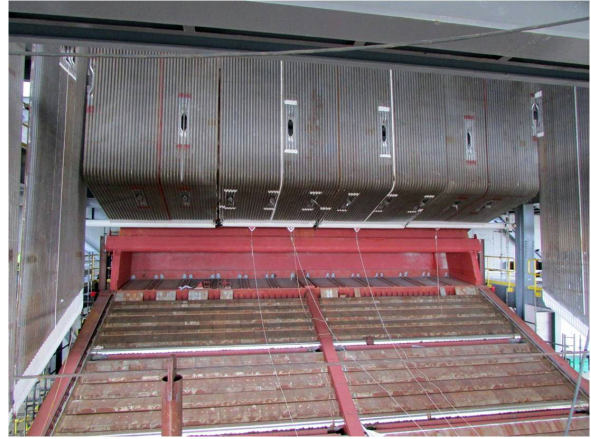
A view inside the furnace shows the fuel ram feeder, DynaGrate wave moving grate combustion system, and weld overlay for lower furnace tube corrosion protection.
