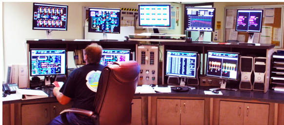
Based on a successful 20-year operating history, SWA extended the operations and management contract through 2018.
