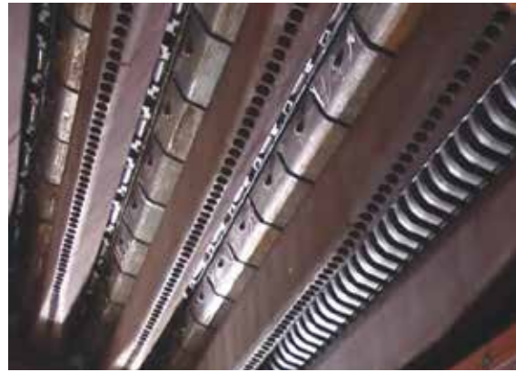
Below the grate: No flex tubes below the grate
