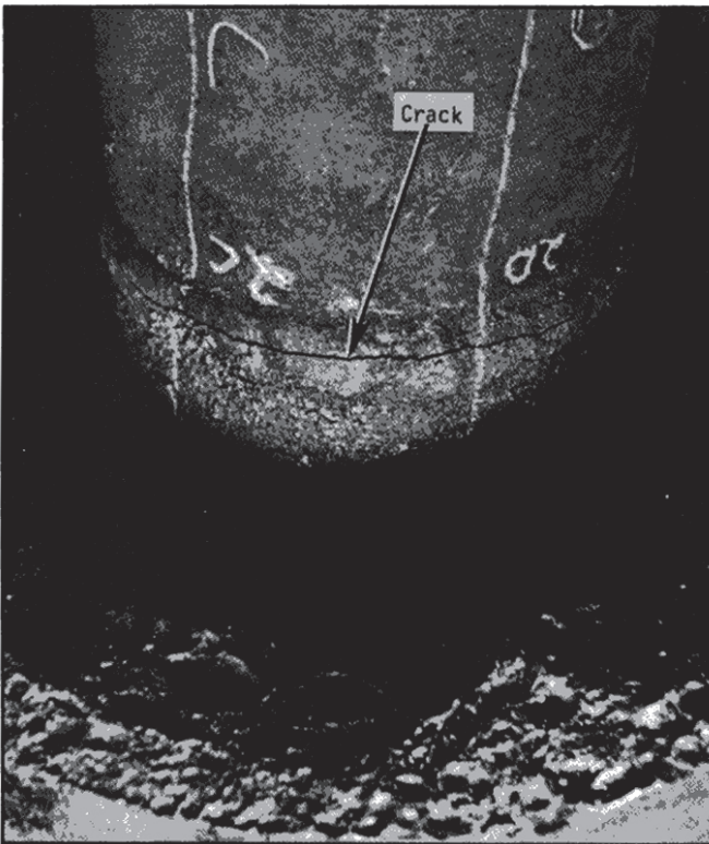
Figure 4 Dissimilar weld cracks.
